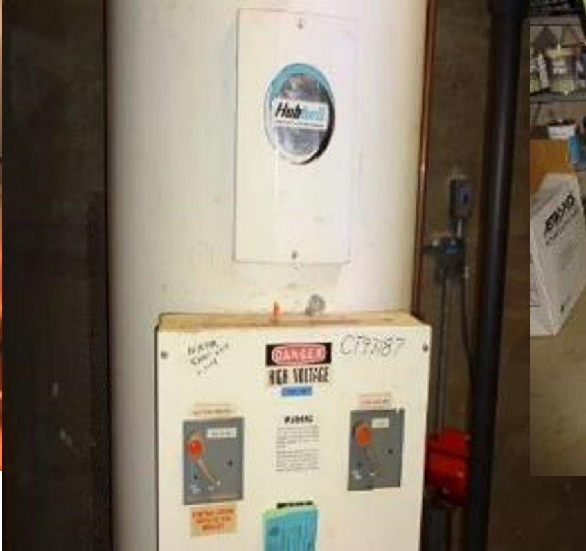
Original water heater – 1975
